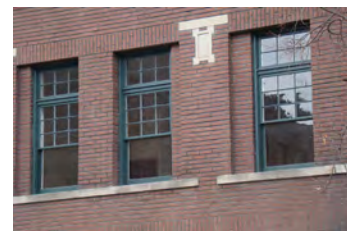
Operable windows can help reduce energy bills by facilitating air circulation from the exterior to the interior.
