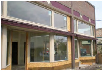
Retractable awnings and recessed entranceways provide several energy efficiency benefits.
